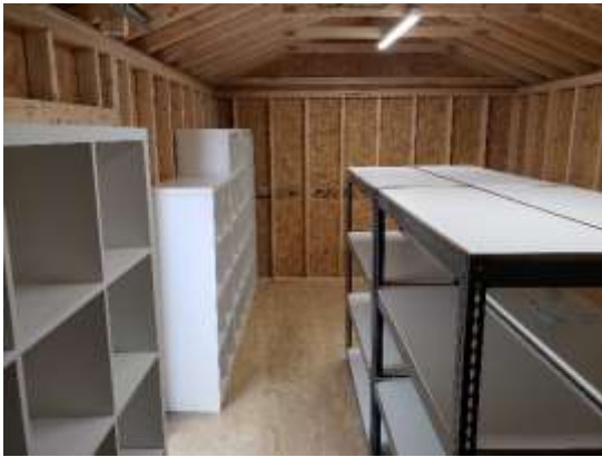
Shelving units, electricity + lights
